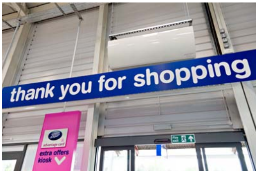
Over door heaters at Boots UK's store in Sovereign Retail Park, Eastbourne
